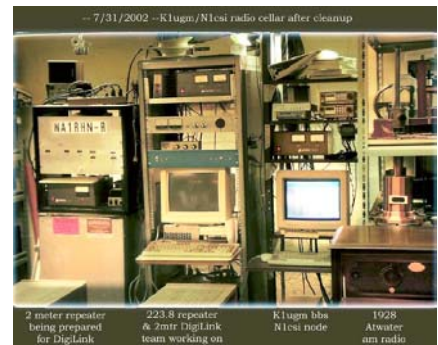
2 mtr rpt for digi-link 220 rpt for UGM pkt station 1928 Atwater AM radio
