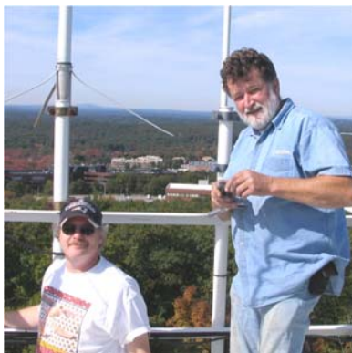
Lou N1UEC and Joe K1LBG Installing our new Super Station Antenna, Ted K1QAR is the guy "behind" the camera.
